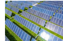
Solar PP 50 MW at Kaltim
